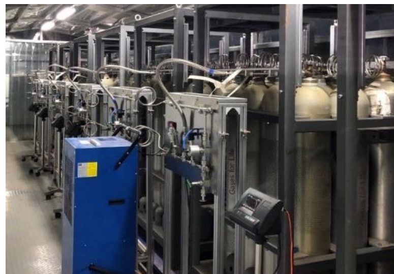
Gas storage system
